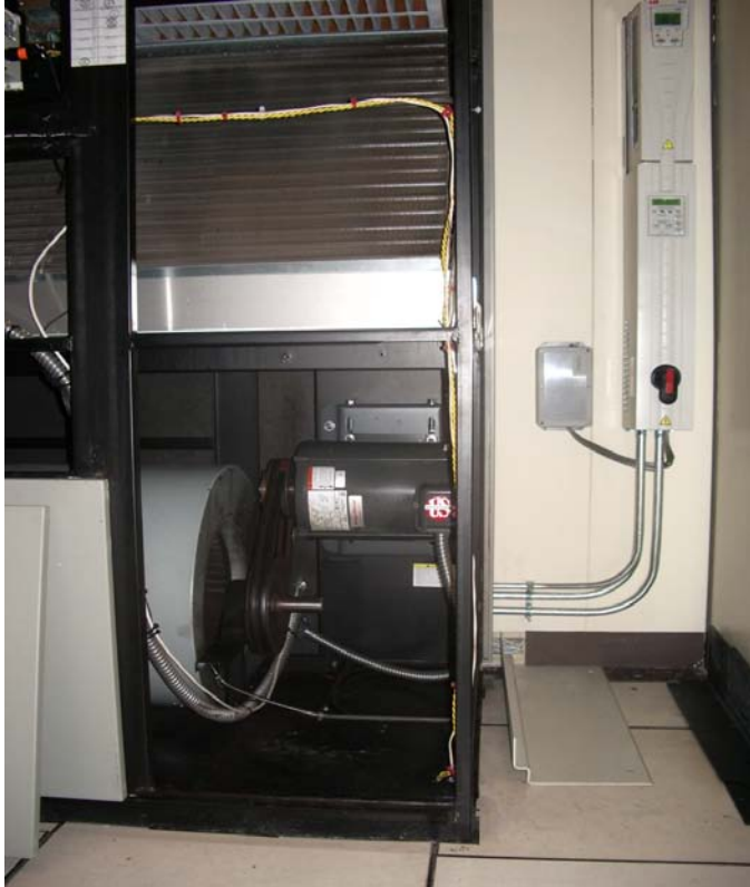
Figure 3. VSD installation: VSD with bypass mounted on wall near the CRAC (Credit: Symanski 2012).
