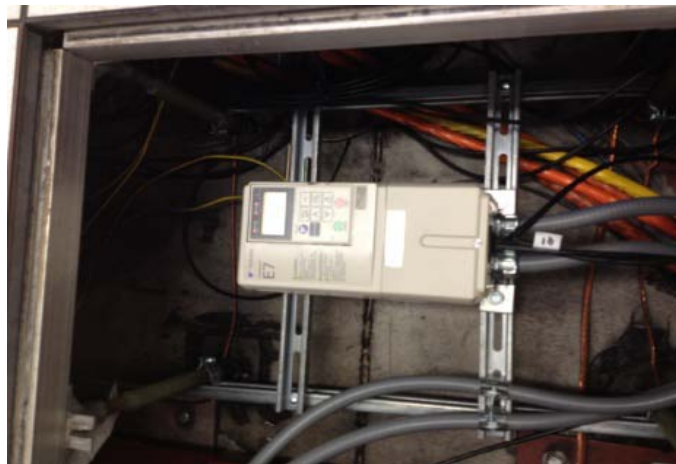
Figure 4. VSD installation: plain VSD mounted under the floor near the CRAC (Credit: Ritenour, 2012)
